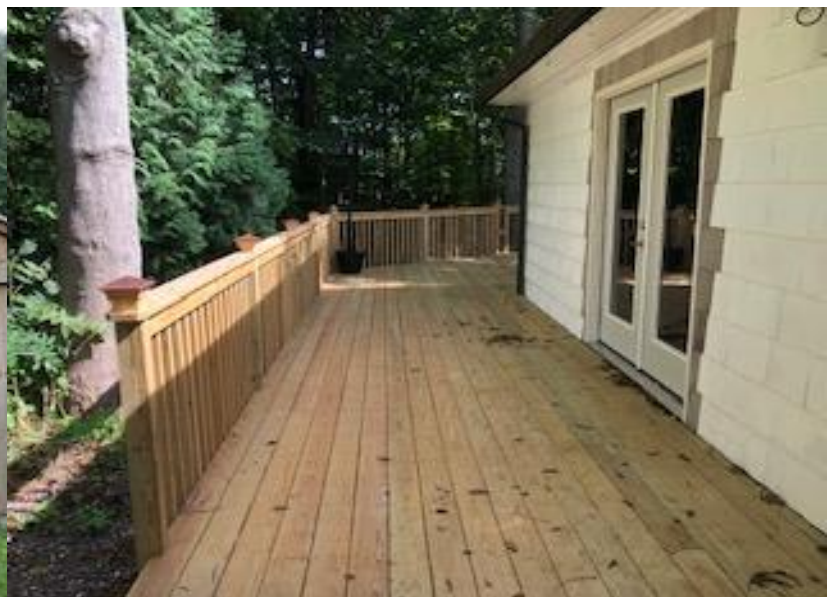
Our new deck surrounds the Nature Lab thanks to Mayor Stewart and the City of New Britain!
